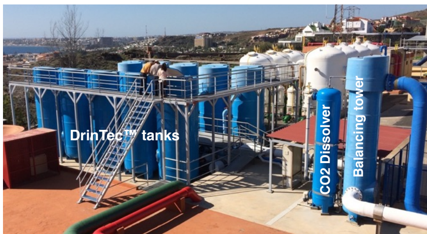
Fig. 1.3: General overview of ten DrinTec™ limestone contactors installation with CO 2 low pressure dissolver.
