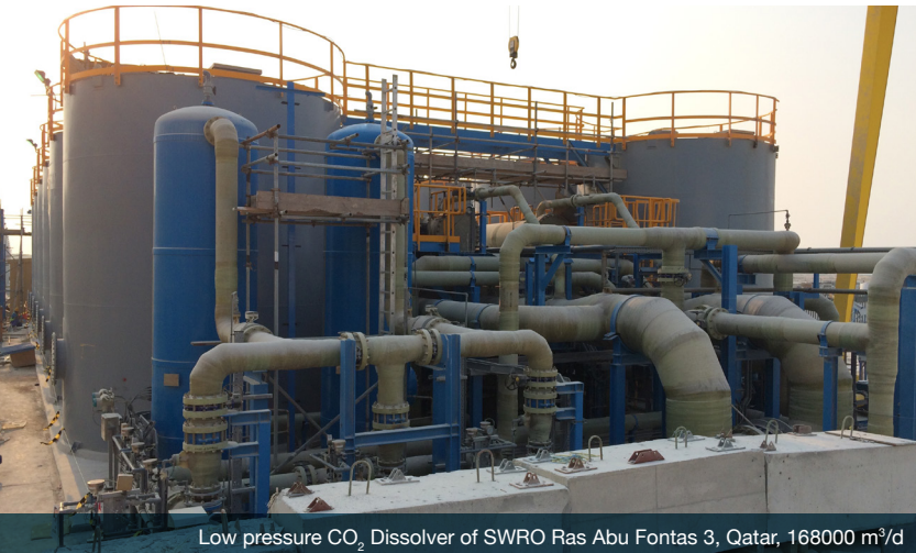
Low pressure CO 2 Dissolver of SWRO Ras Abu Fontas 3, Qatar, 168000 m 3 /d
